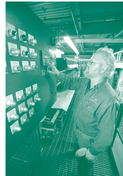
Robert Armstrong, GHU Water Treatment Plant employee, operates the filter press controls.
