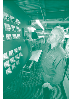
Robert Armstrong, GHU Water Treatment Plant employee, operates the filter press controls.
